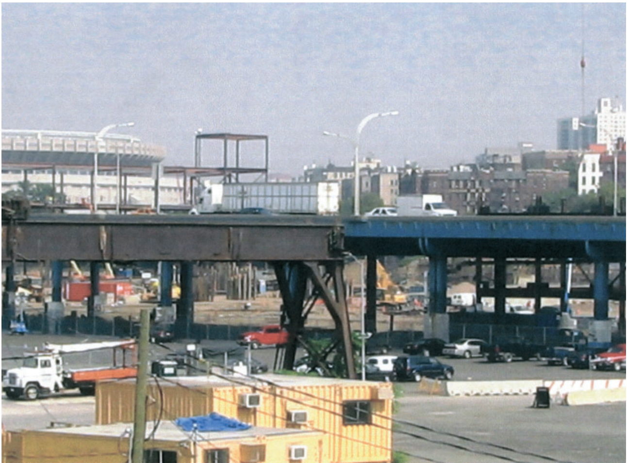
Figure 11. Early construction at Gateway, September 21, 2007. The original Yankee Stadium (rear left) is still standing and the Bronx Men's House of Detention has been completely demolished. The elevated blue roadway is the Major Deegan Expressway adjacent to Gateway. Today the parking lot pictured in the foreground is used for outdoor events.
